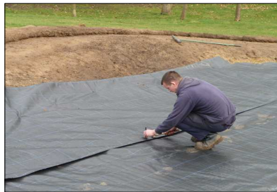
A new membrane goes in an 18th fairway bunker to prevent gravel rising to the top of the sand
