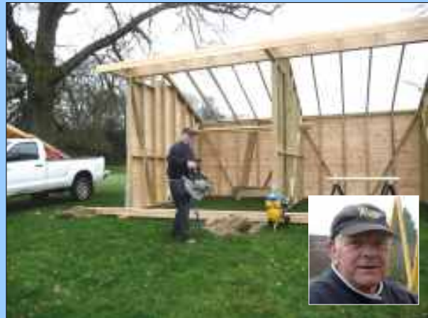
Jim Thorpe constructing the all-weather driving booths that he generously donated to the Club
